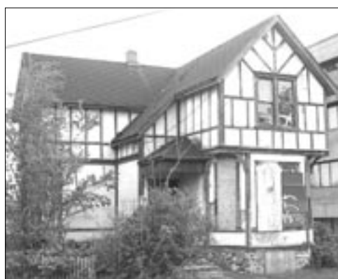
1909 Birch - Boarded up for at least 20 years - roof now has holes in it.
